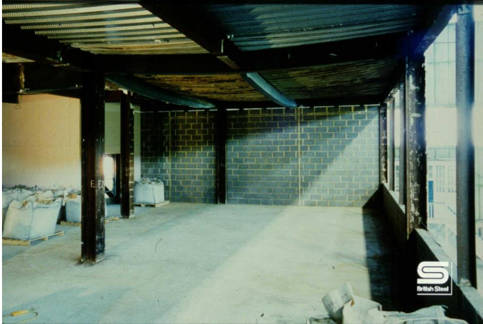
Deformation of the hot part of the floor
