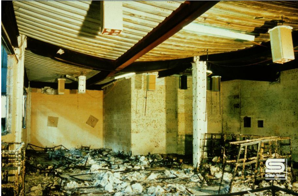
Deformation of the hot part of the composite floor
