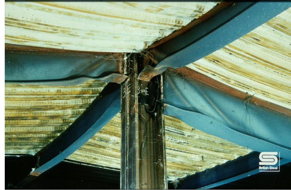
Deformation of metal elements in the right of a protected column
