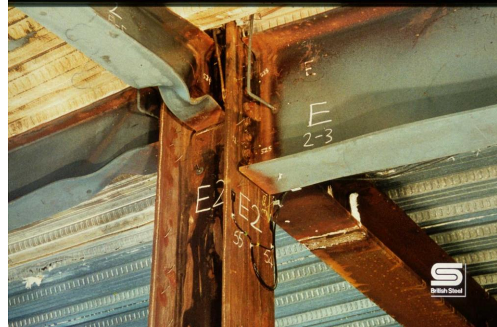
Deformation of the metal elements around the protected column
