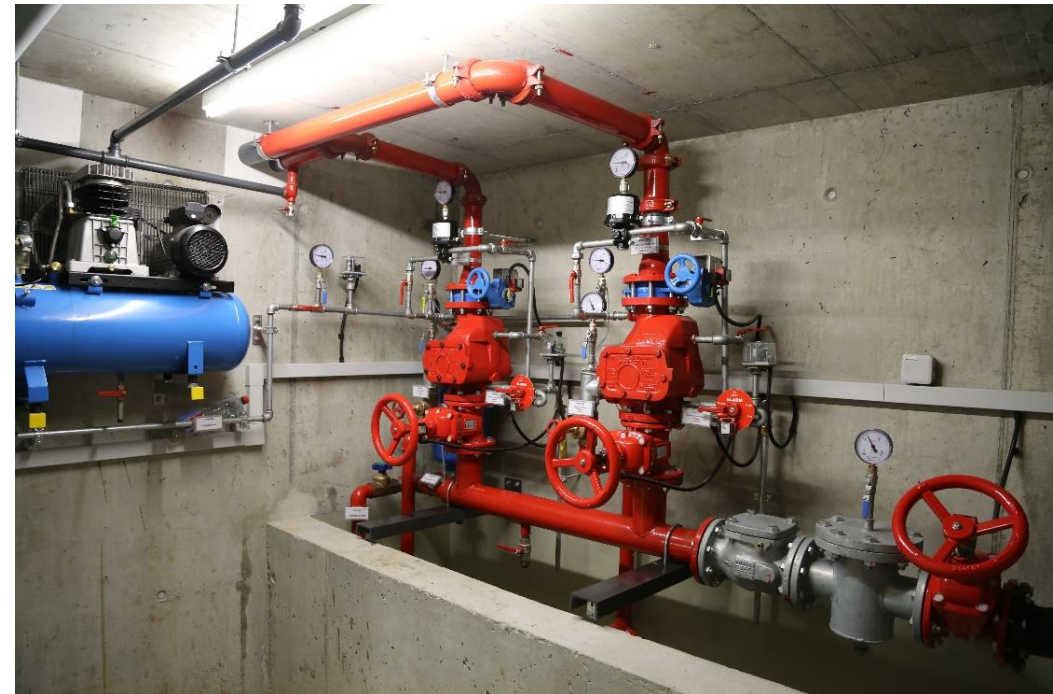
Underwater installation (risk of freezing)
